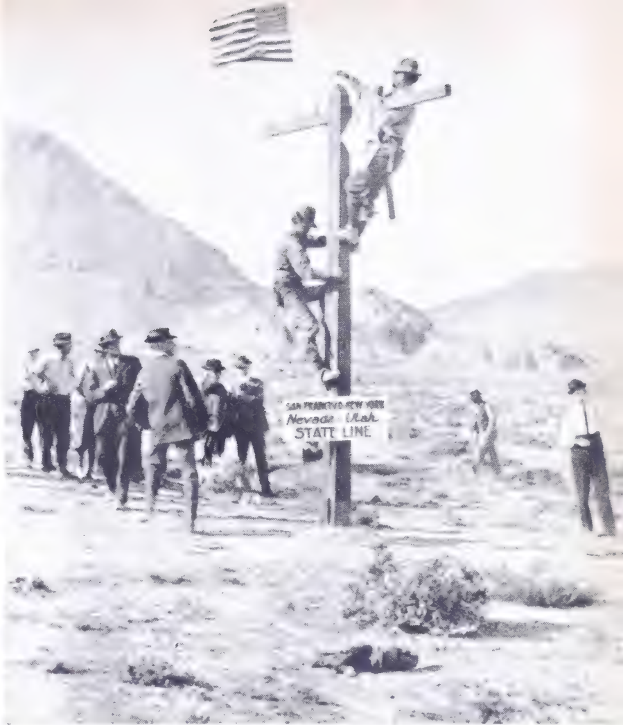
The first open wire line (linked here at the Nevada-Utah border) could carry only three calls and was vulnerable to interruptions.
